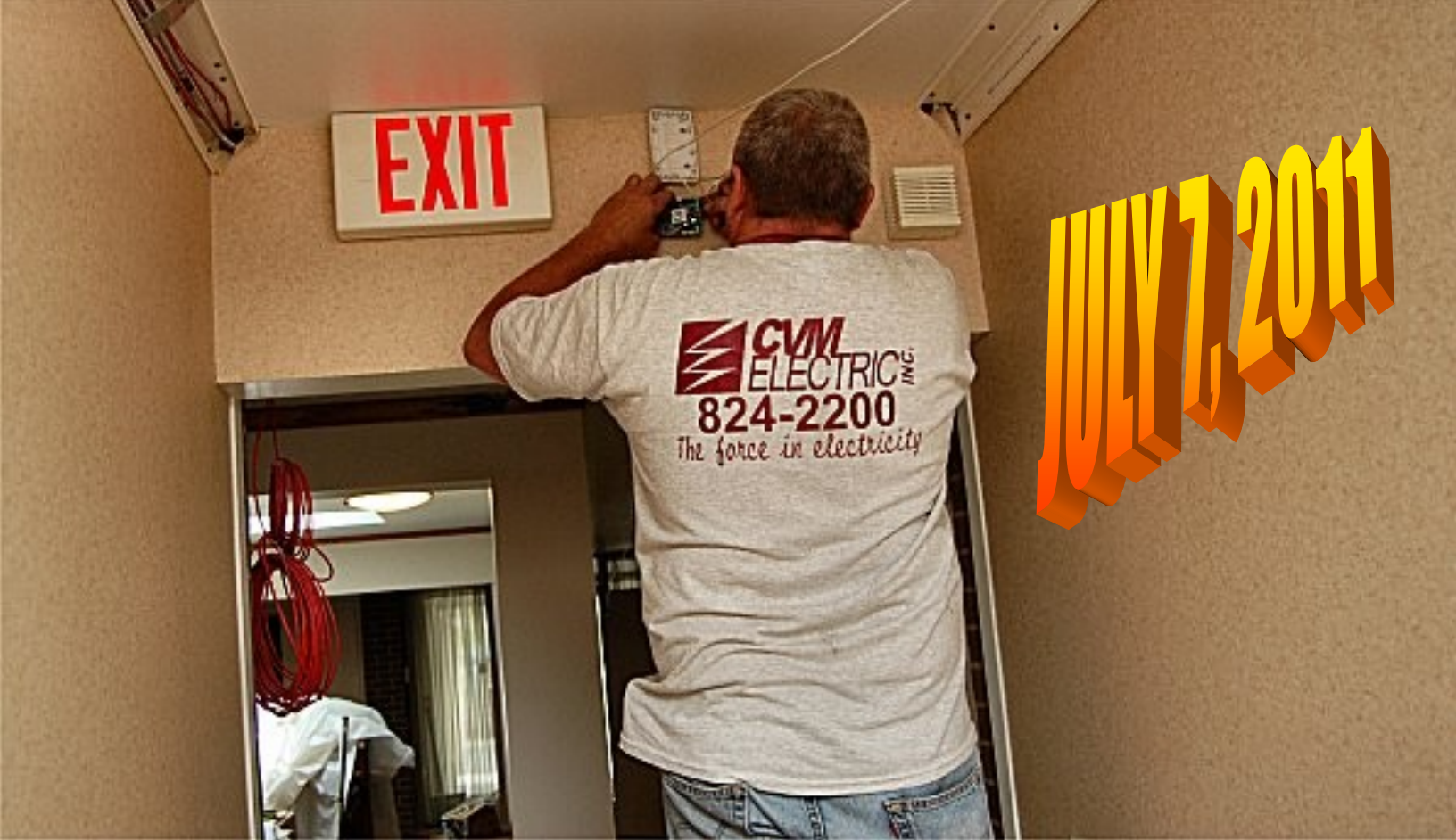
MOTION SENSOR INSTALLATION
